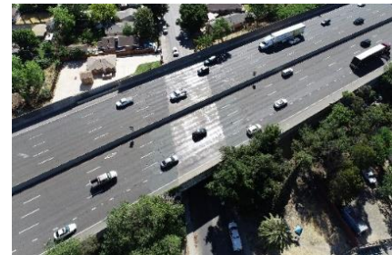
Crews are schedule to replace the bridge deck on SR-99 at 21 st Avenue during the four-day closure.
