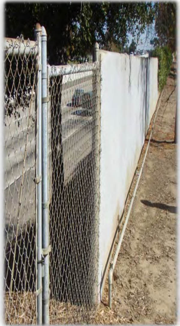
Figure 4 - Existing SW- "SW16" overlaps a 6 ft x 1,062 ft experimental SW composed of shotcrete on chain link fence. This is one example of existing barriers that is proposed to be replaced to match the overall proposed SW aesthetics and service life.
