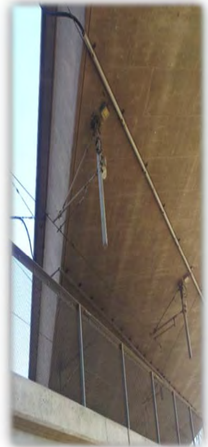
Figure 2 – RT Light Rail Conflict The RT messenger line is connected to soffit of Brighton OH Br. No. 24-0289R.
